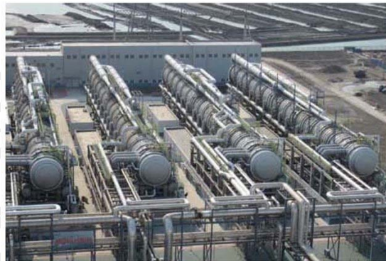
Figure 4. Parallel IDE MED units, 4 x MED 25,000 \text{ m}^3/\text{day} Units, Tianjin, China.
