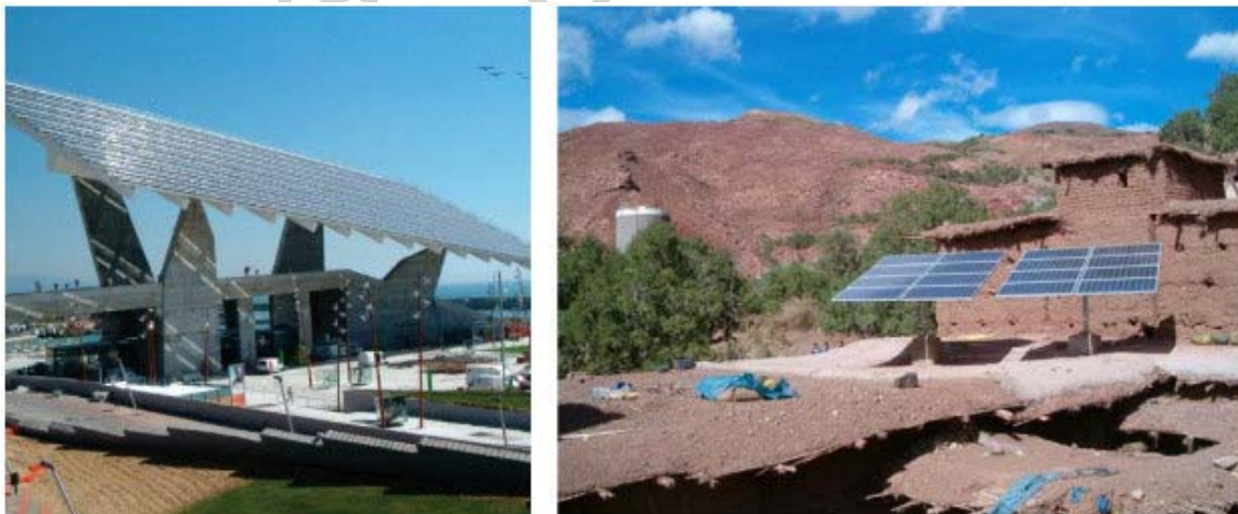
Figure 1: The photovoltaic pergola in Barcelona's Forum of the Cultures (left) and the generator for a pumping system in Morocco (right)
