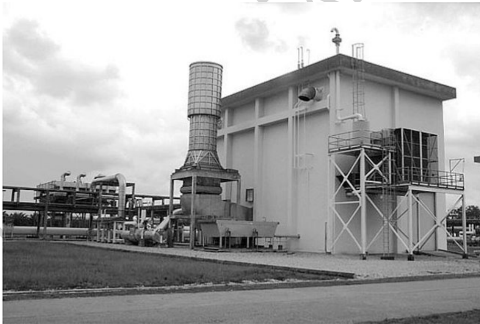
Figure 1 – An Example of a Compressor Station
